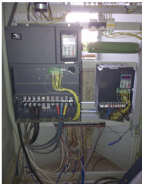
Fig. 9 Power cabinet of wire drawing line
