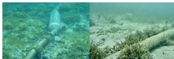
Fig. 1. Photographs of underwater electrical cables.
