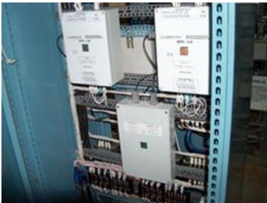
Figure 5. LIRA device in a 110 kV substation
