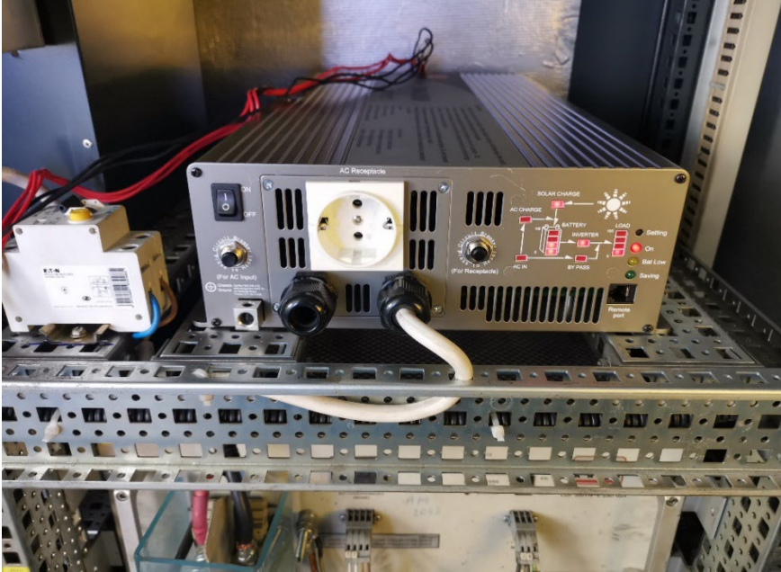
Fig. 7. View from the appliance block with the controller connected to the solar panels.
