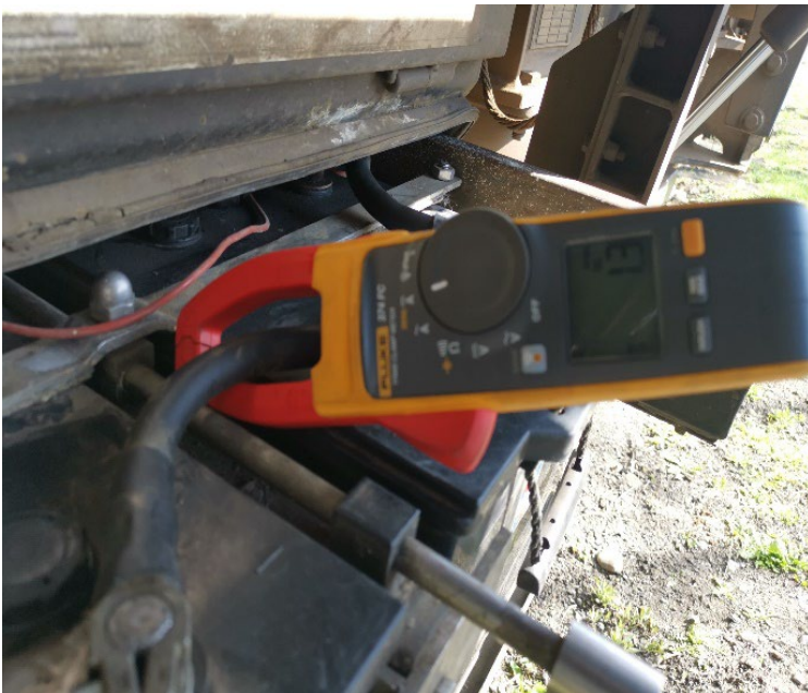
Fig. 8. Measuring the charging current of the battery pack with the ammeter clamp measuring device.
