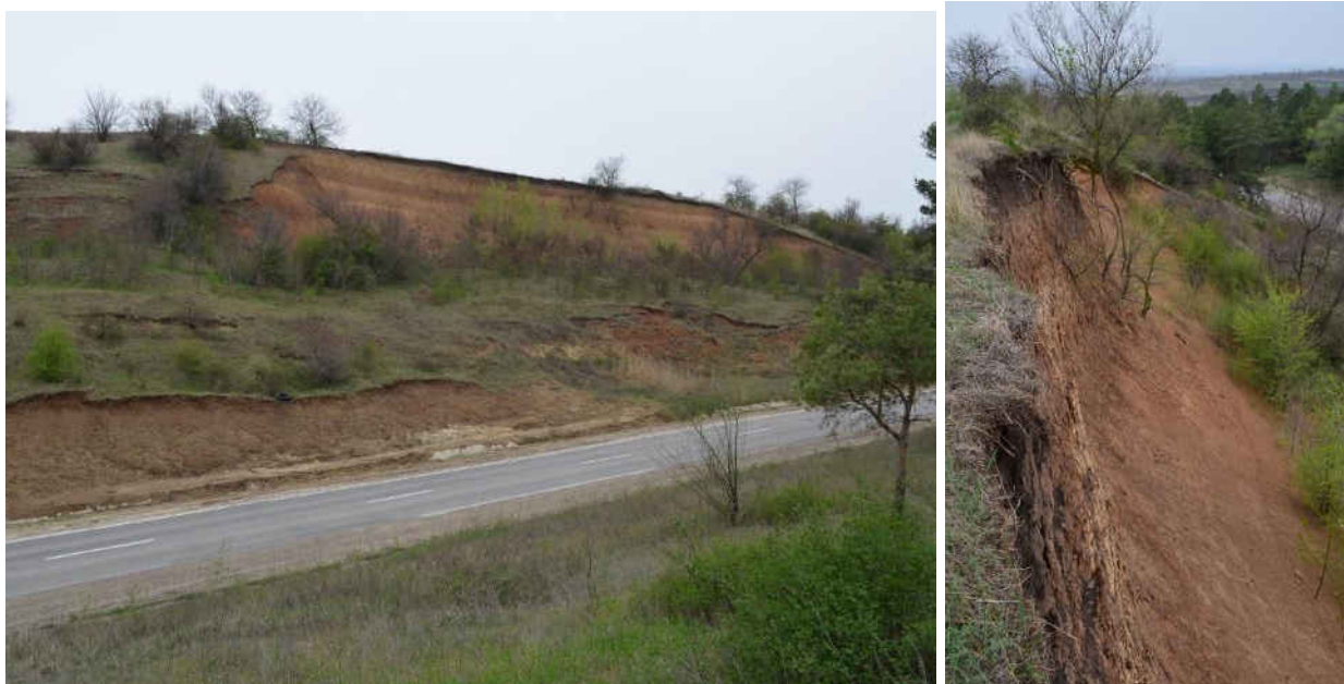
Figure 2. Deformation of the left slope of the deep excavation at PC1441+00 of the M21 road, Brest-Chisinau-Poltava Foto: Cîrlan Alexandru, April 2017.
